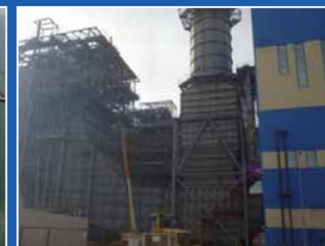
Banha Power Plant, Egypt
